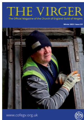
Colin Campbell inspecting the roof of St Mary's Episcopal Cathedral, Edinburgh (see page 4)
